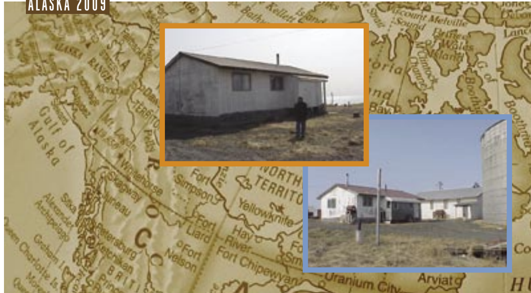
The parsonage and church in Shaktoolik, Alaska, are examples of buildings that will benefit from NWC sponsorship.
